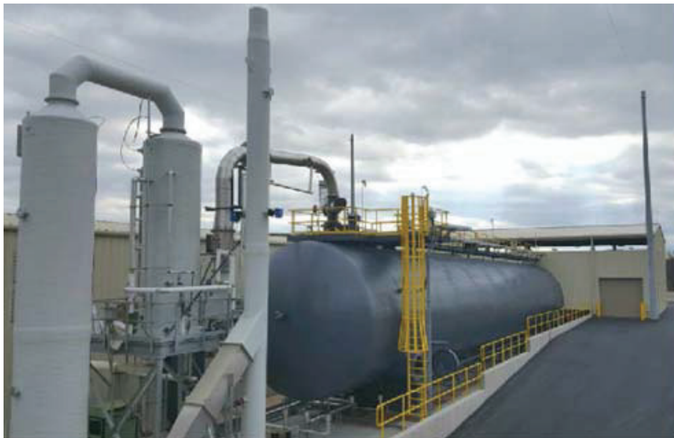
FIGURE 4.2 Ammonium Perchlorate Rocket Motor Destruction Facility thermal treatment chamber. SOURCE: R. Hayes, president, El Dorado Engineering, “El Dorado Engineering’s Technologies for the Demilitarization of Conventional Munitions,” presentation to the committee, October 24, 2017.
