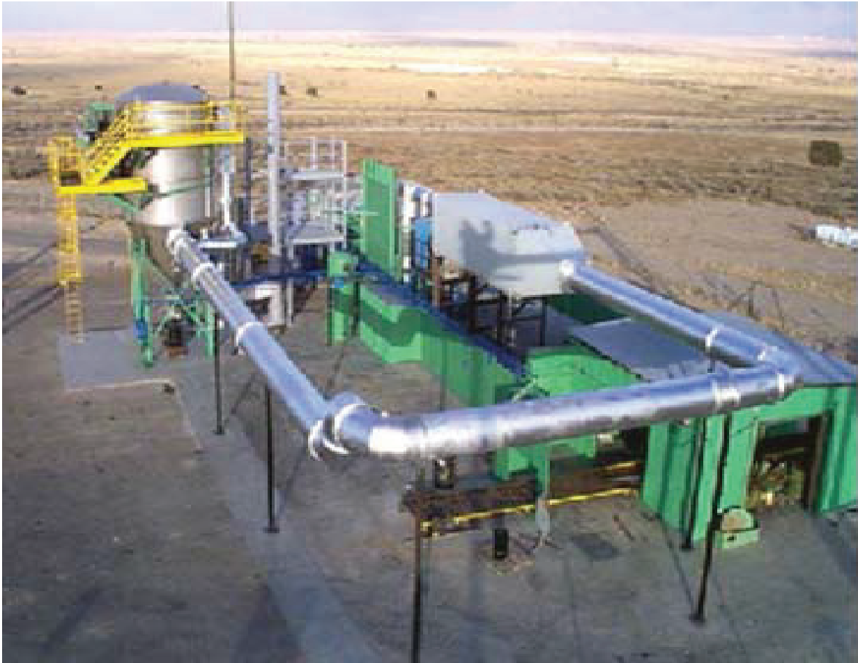
FIGURE 4.5 APE 1236M2 and pollution abatement system. SOURCE: J. McFassel, product director for demilitarization, PEO AMMO, and O. Hrycak, chief engineer, Office of the Product Director for Demilitarization, PEO AMMO, “Emerging Technologies Addressing Alternatives to Open Burn and Open Detonation,” presentation to the committee, August 22, 2017.
