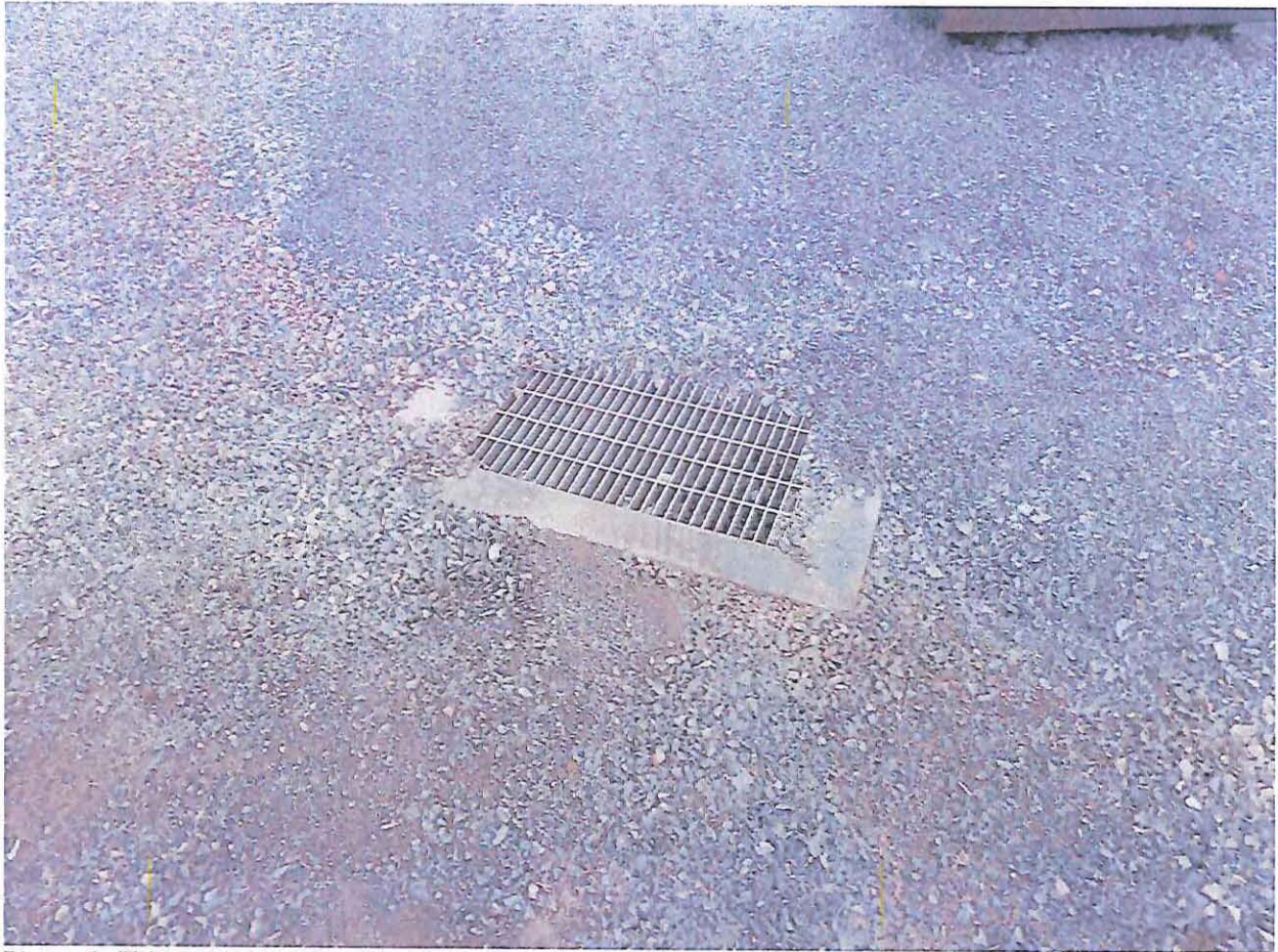
Picture 5: Holston Army Ammunition Plant – December 9, 2015 at 4:00 P.M. Storm water collection point near Pan 3 of the permitted Burning Ground. – Picture taken by Javier Garcia.
