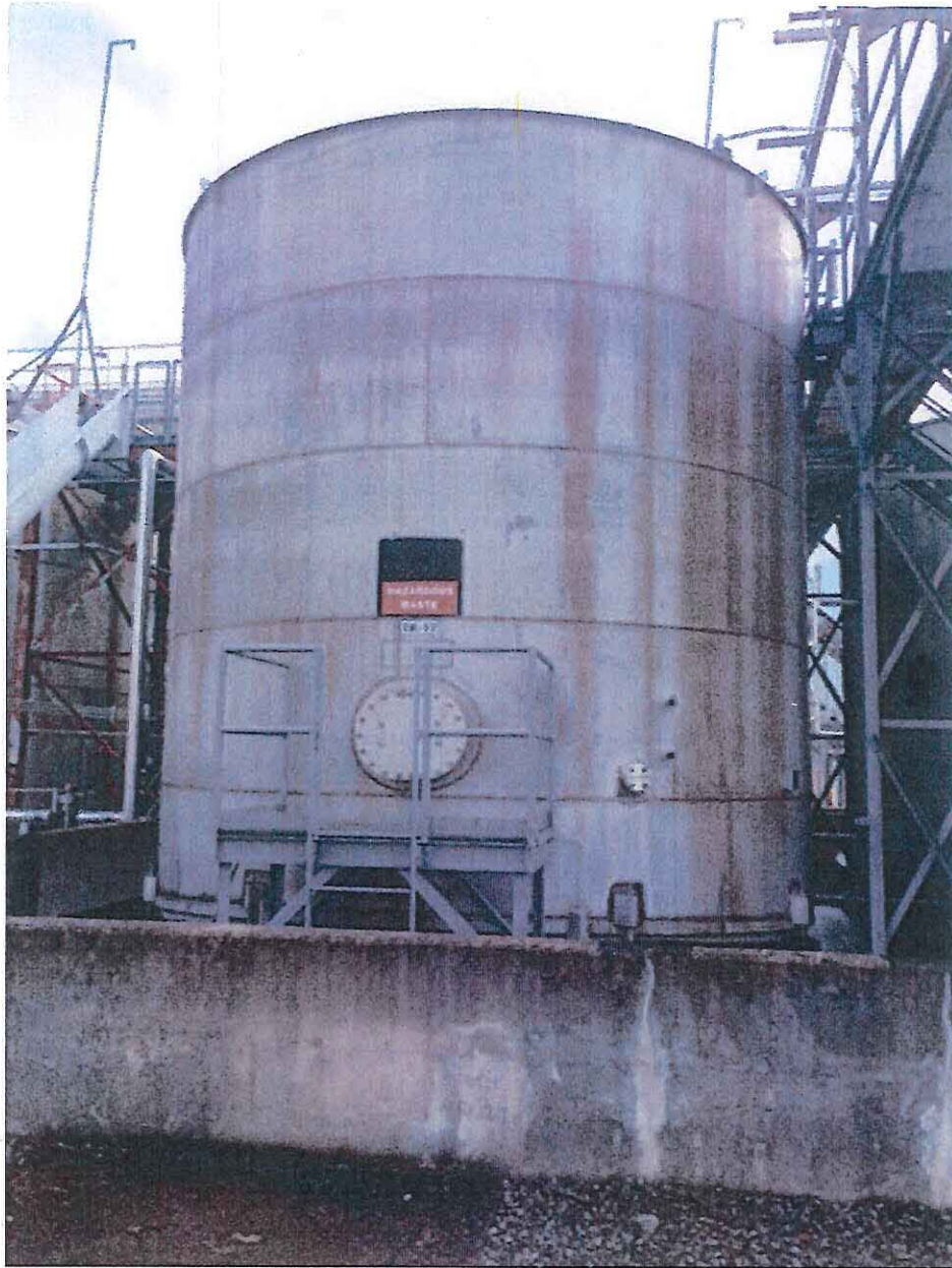
Picture 10: Holston Army Ammunition Plant – December 10, 2015 at 10:37 A.M. Side view of hazardous waste storage tank designated as Tank 17 showing required “Hazardous Waste” marking. Picture taken by Javier Garcia.
