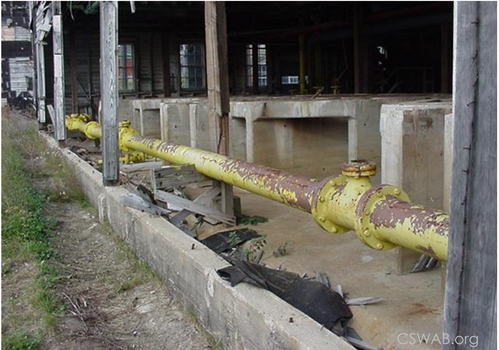
PCB bulk waste > 50 ppm. Dried applied paint as high as 22,000 ppm.
